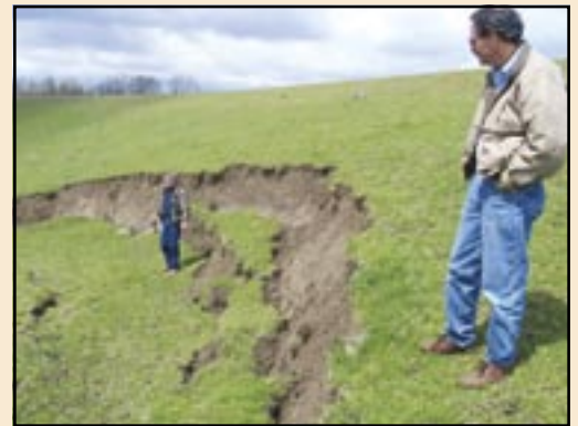
Eddie Stewart and Pete Montalbano of the Vicksburg District Corps of Engineers inspect a slide at Station 2819 in Bolivar County, MS.
